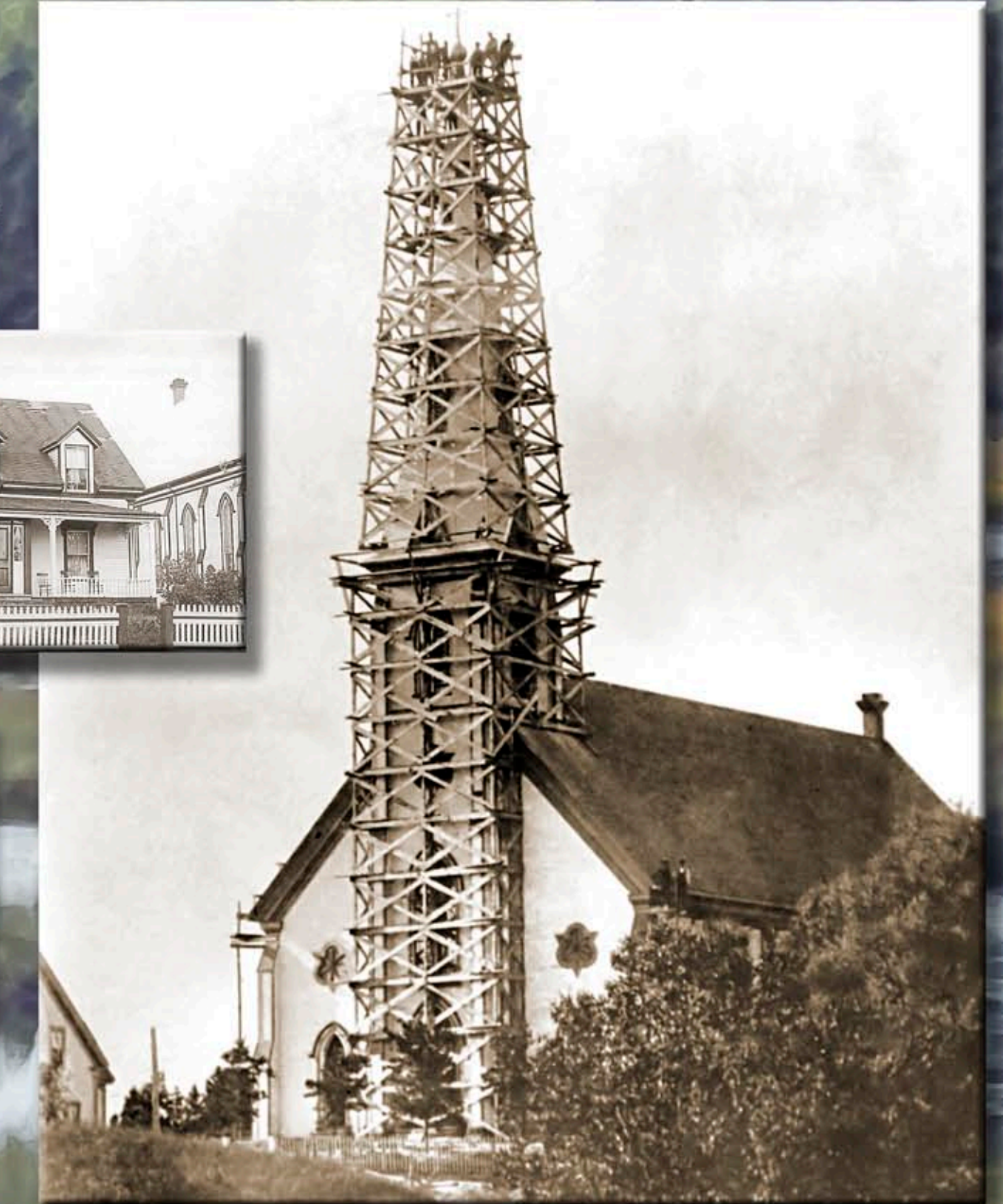
Repairing the church steeple after being struck by lightning, 1919-1921. When St. Mary's Church opened in 1897, it could hold 1,000 people.
